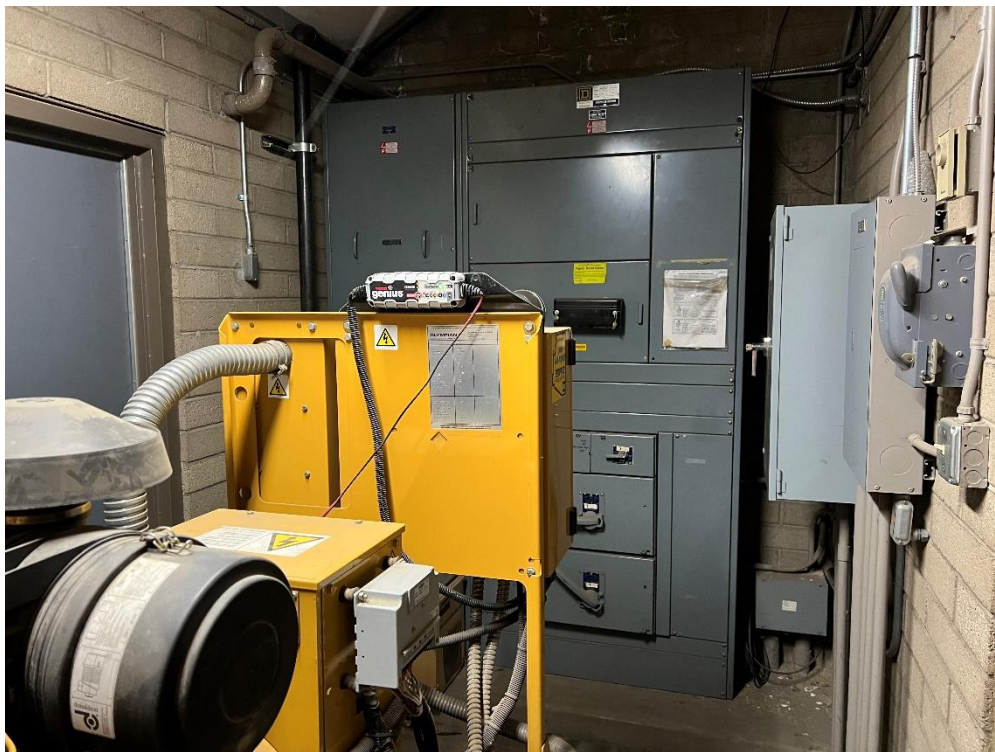
Sub-panel. Tower room is behind locked door to left.
